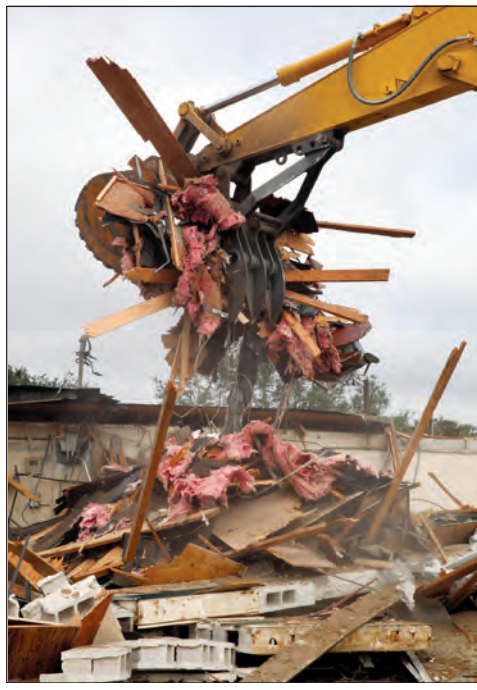
The Stone Beads building, which has stood on the Brighton site since the 1960s, is demolished by an excavator Feb. 5.
