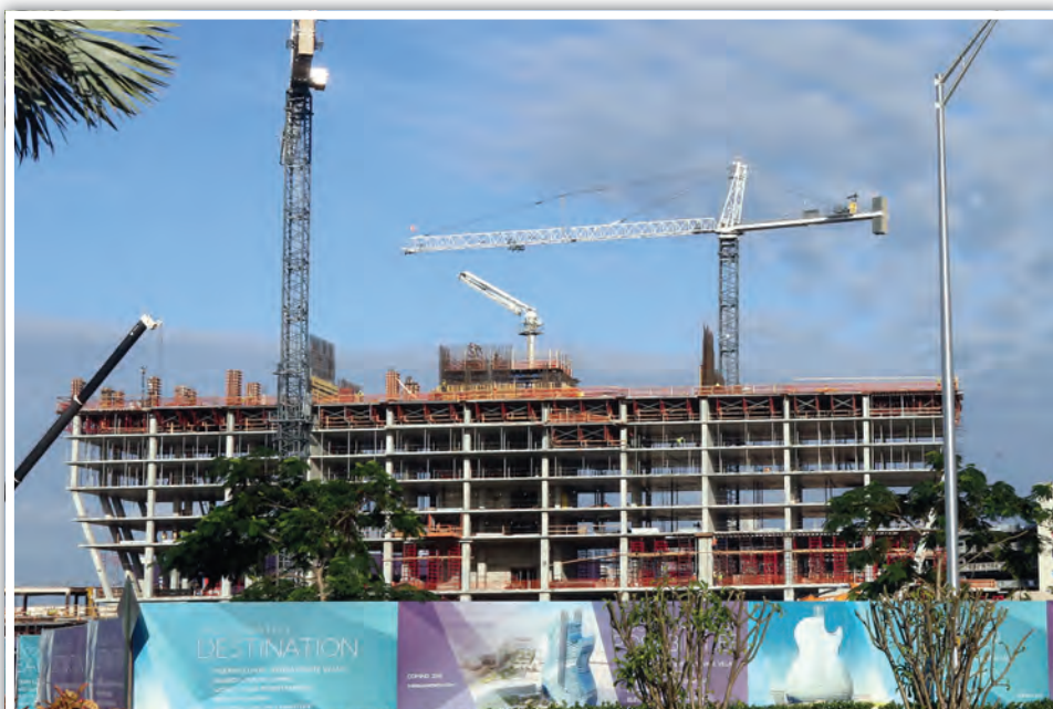
TAKING SHAPE: Here's the view on Nov. 16 of the guitar hotel under construction at the Seminole Hard Rock Hotel & Casino Hollywood. Construction is expected to be completed by mid-2019.
