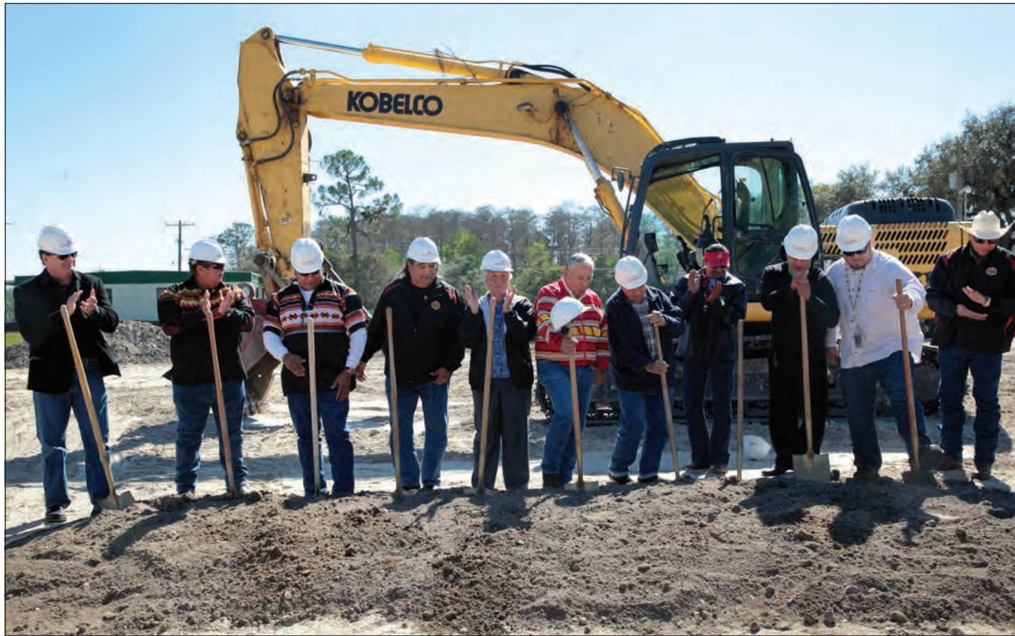
Tribal and construction officials turn the dirt Jan. 28 on the site of the future Big Cypress Medical Center.
